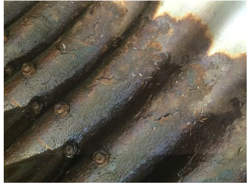
Pitting & Flaking of Floor
